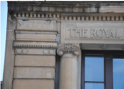
Front Façade: Detail of the Entrance, Showing Damage to the Entablature and Columns, Probably due to Water Infiltration
