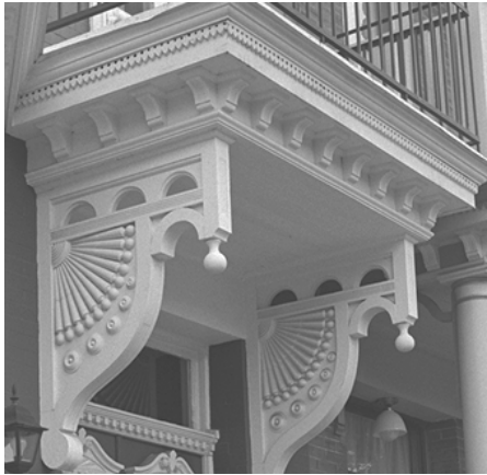
Woodwork deterioration sometimes looks worse than it is. Often minor repairs and repainting are sufficient.
